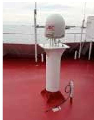
Inmarsat-F Antenna wire was cut
