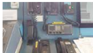
VHF1 handset was removed.
